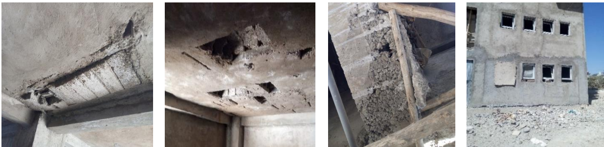
Figure-1 Poor execution of ribbed slab and Poor quality of columns which is due to less vibration and formation of cracks on a plastered surface. (Source: Touristsite condominium, Megenagna).
